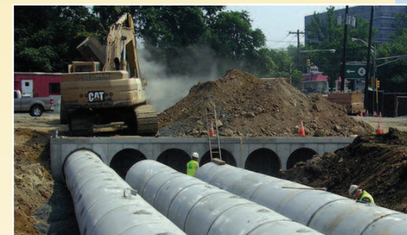
Underground storm water storage
